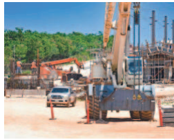
Contract personnel and heavy equipment can be seen as work continues along a roadway, just past the turnoff to the Guam National Wildlife Refuge, on March 31. The roadway is being installed near Ritidian Point to allow easier access to an area designated for several live-fire training ranges.
