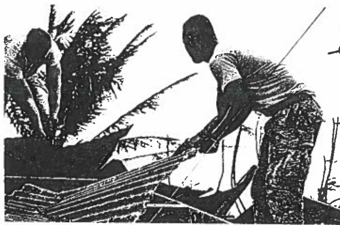
ROOF WORK: Soldiers and airmen from Task Force Engineer remove damaged roofing at a home on Saipan on Monday. Task Force Engineer is providing much-needed temporary roofing to the island's residents, who are still recovering from Super-typhoon Yutu. Military service members from Joint Region Marianas and the Indo-Pacific Command are working with the Federal Emergency Management Agency and CNMI officials to recover from the storm's devastating impacts. Sgt. 1st Class Wynn Hoke/U.S. Army
